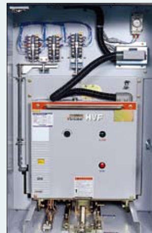
Circuit Breaker in the 'Service' Position
